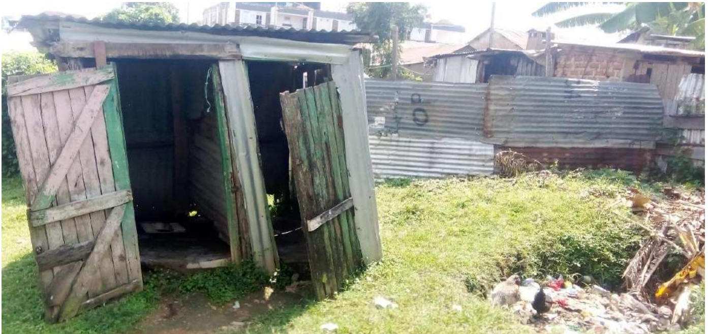
Plate 2 Dilapidated Pit Latrine in an Informal Settlement in Kakamega Municipality
